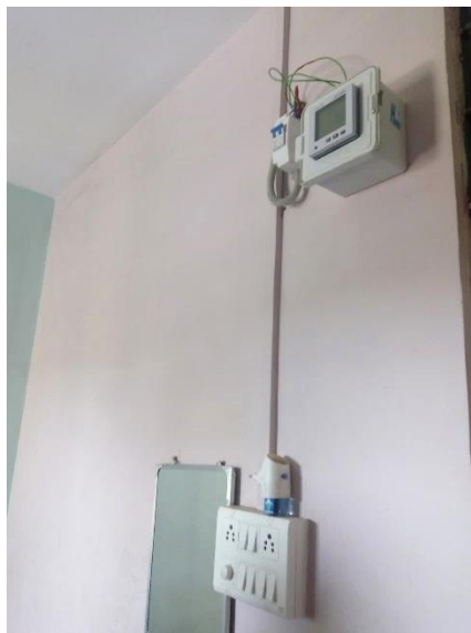
Figure 11 Installed energy meter at dwelling level
